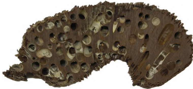
Marine borer damage to a hardwood pylon
