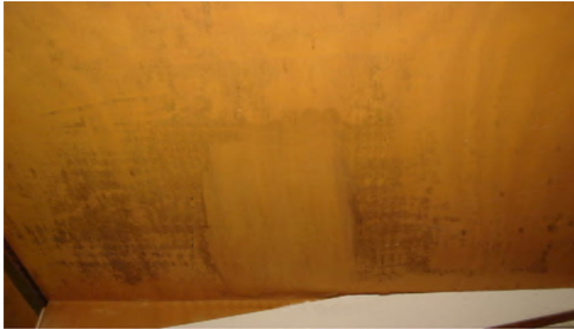
Typical example of surface mould
