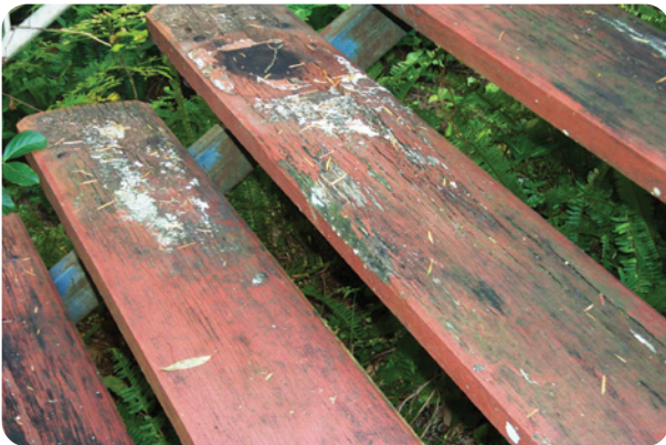
Poor maintenance of stair tread.
