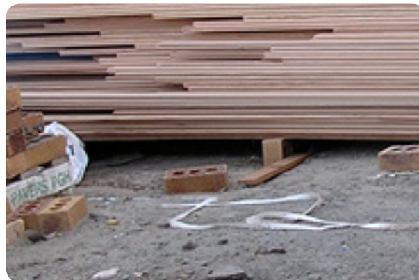
Figure 3.1: Inappropriate site storage can void manufacturer warranties.
