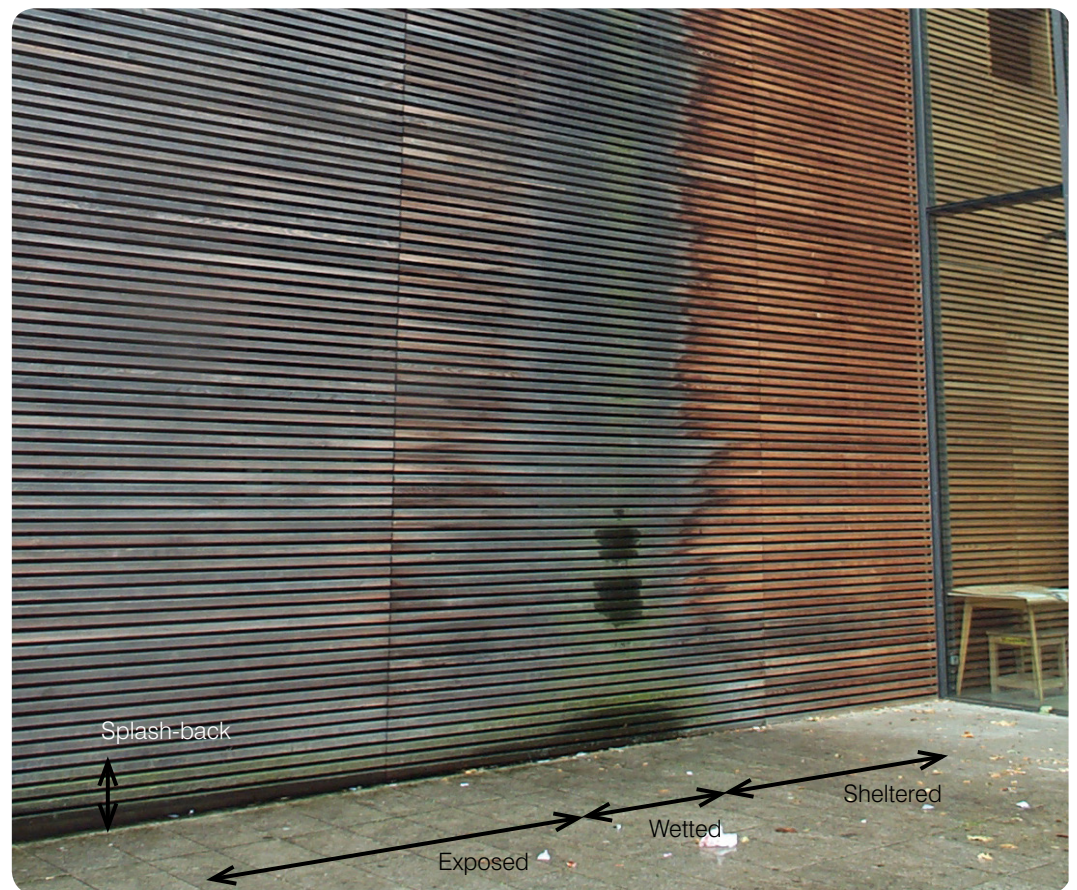
Figure 6: Differential weathering and decay on a facade.
