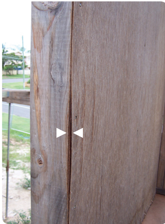
Delamination of plywood sheet bracing (see arrows).
