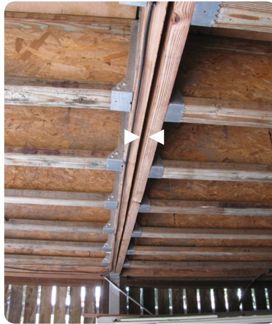
Expansion in flood-affected timber flooring.
