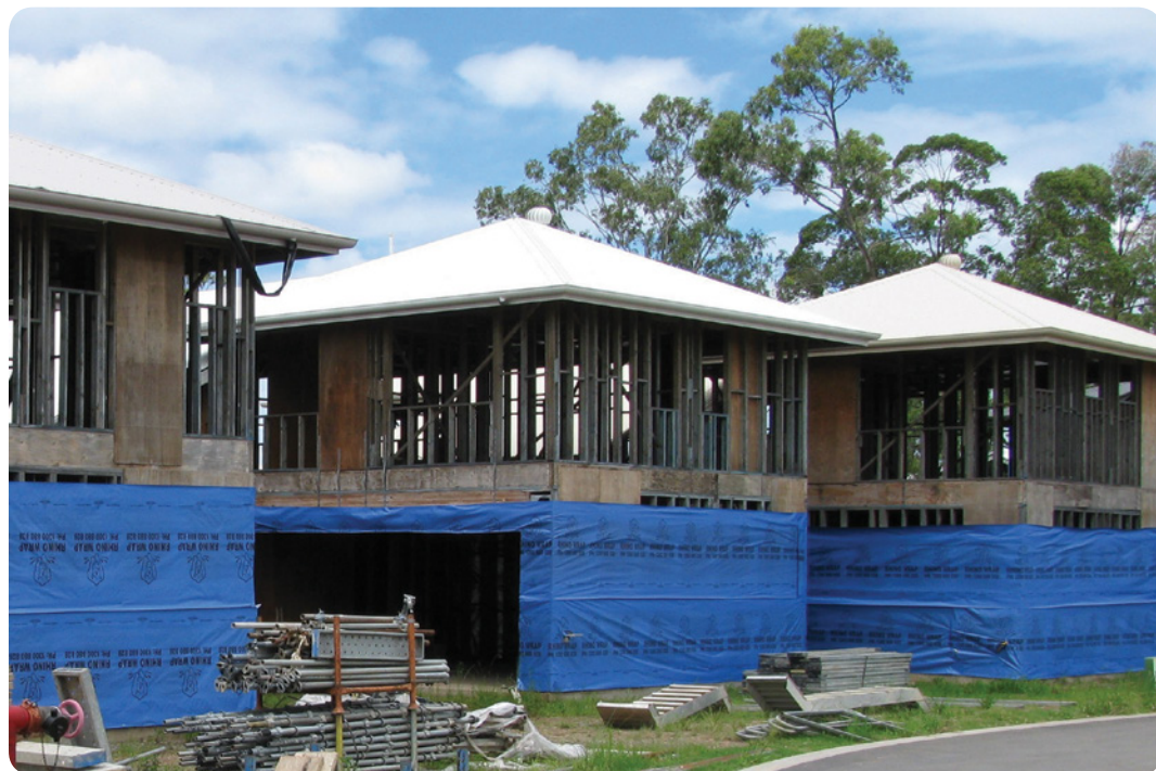
Exposed timber can become discolored and stained.
