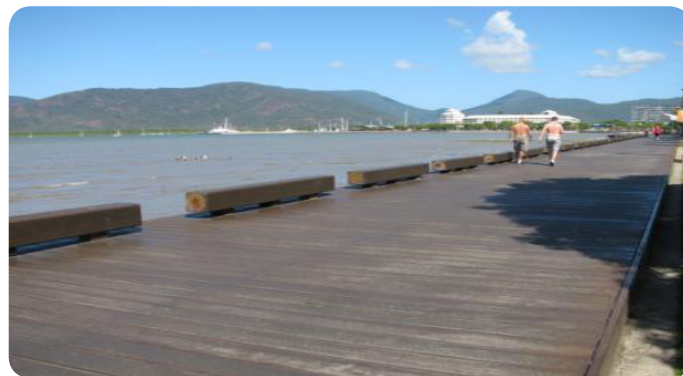
Figure 18: Site-applied pigmented deck stain requiring maintenance.
