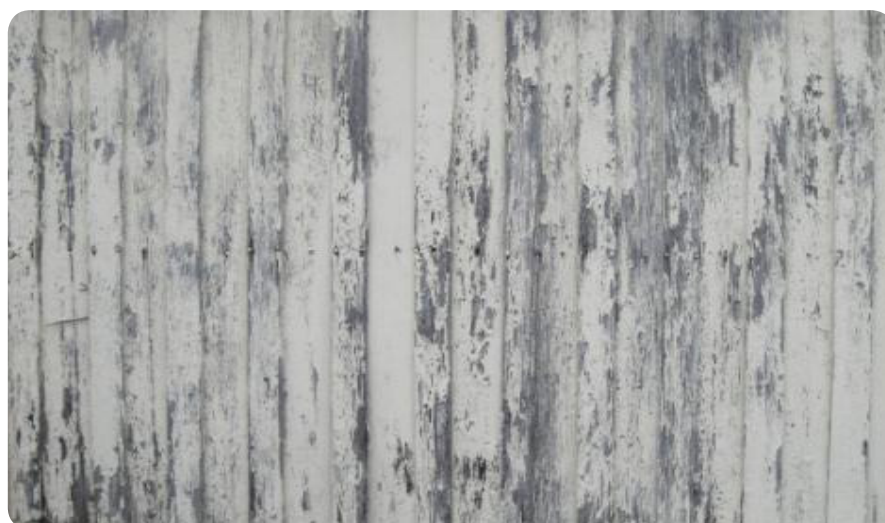
Figure 19: Poorly maintained film-forming finish.
