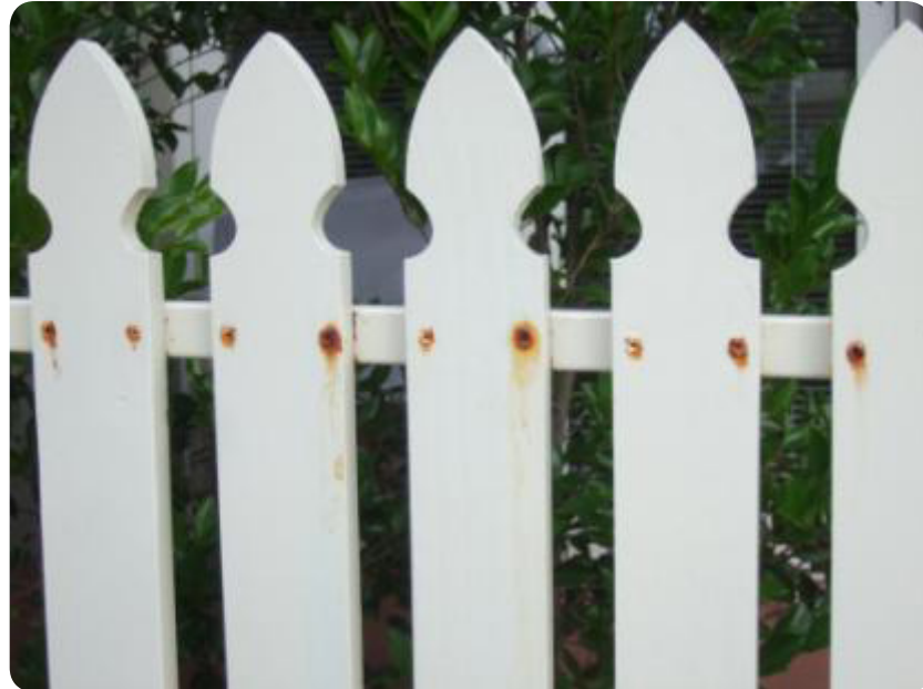
Figure 20: Rapid corrosion of poorly specified fasteners.
