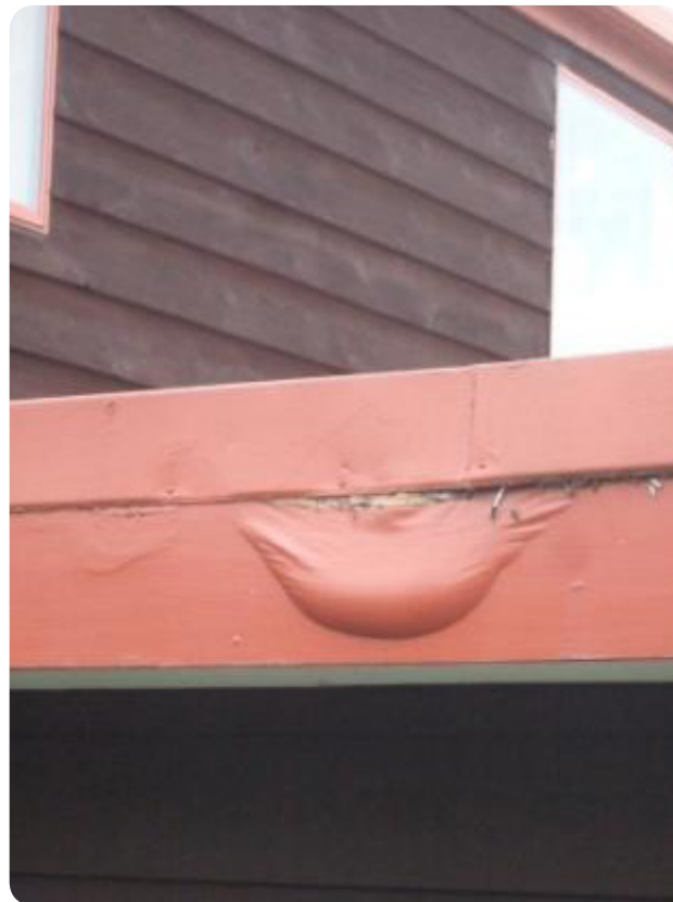
Figure 16: Poorly maintained paint which is trapping moisture.
