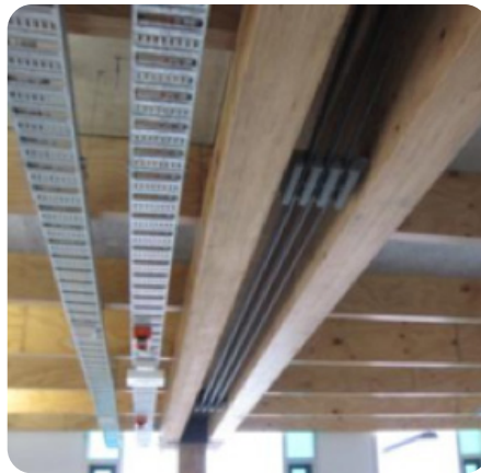
(a) Exposed tendons, no fire resistance.
