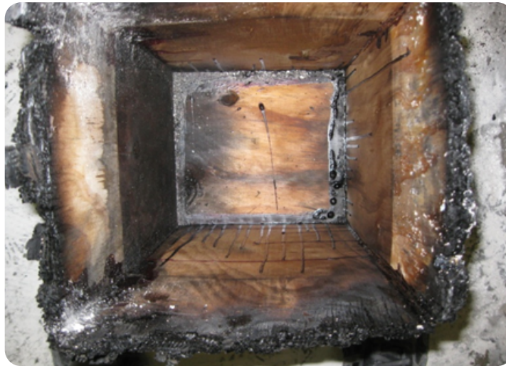
Figure 4.3: Inside a cavity carrying post-tensioning rods, post-fire. 6
