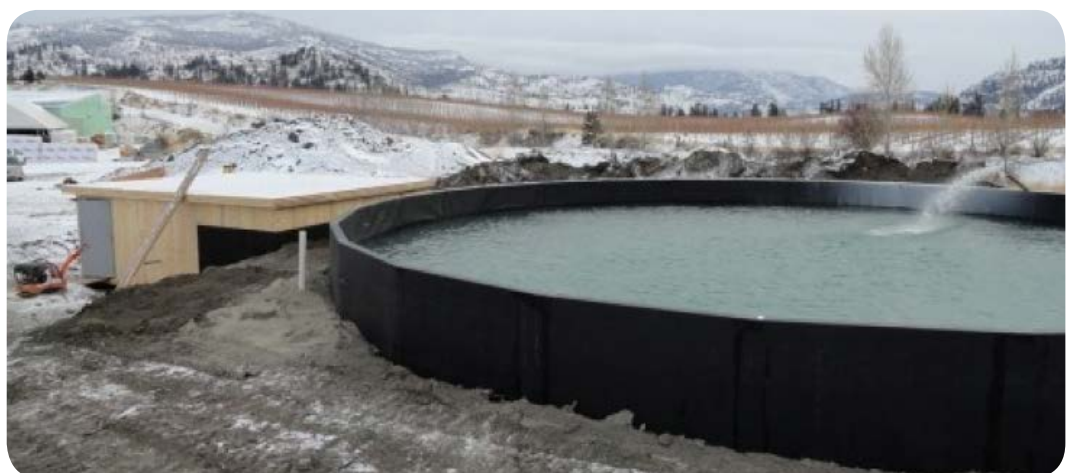
Figure 1.5: Water reservoir. Photograph: Structurlam
