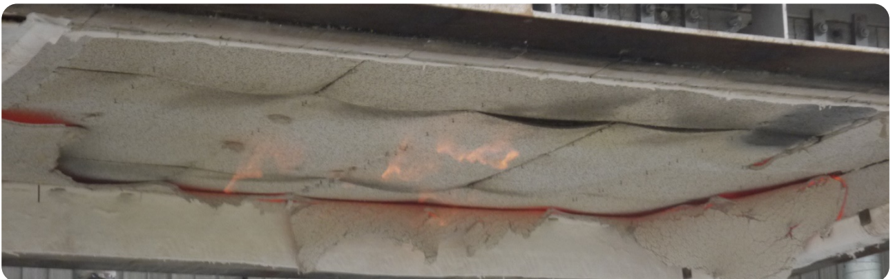
Figure 103: Exposed face showing loss of the face layer of plasterboard and opening of joints in remaining layer.
