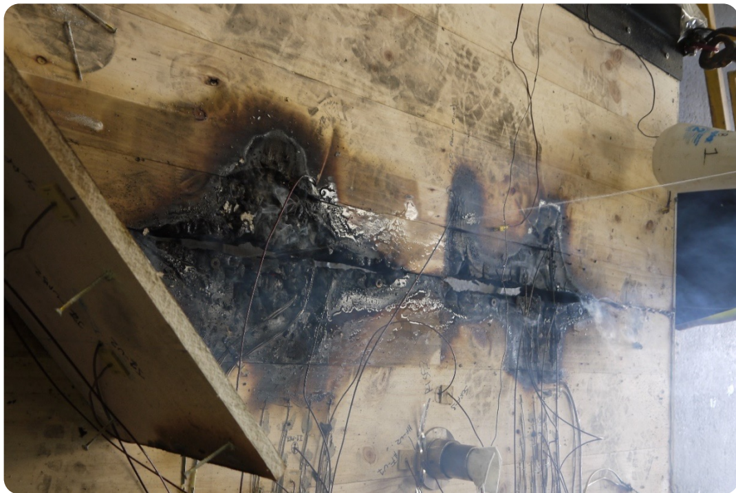
Figure 203: Non-fire side after monitoring period with plasterboard cover removed.
