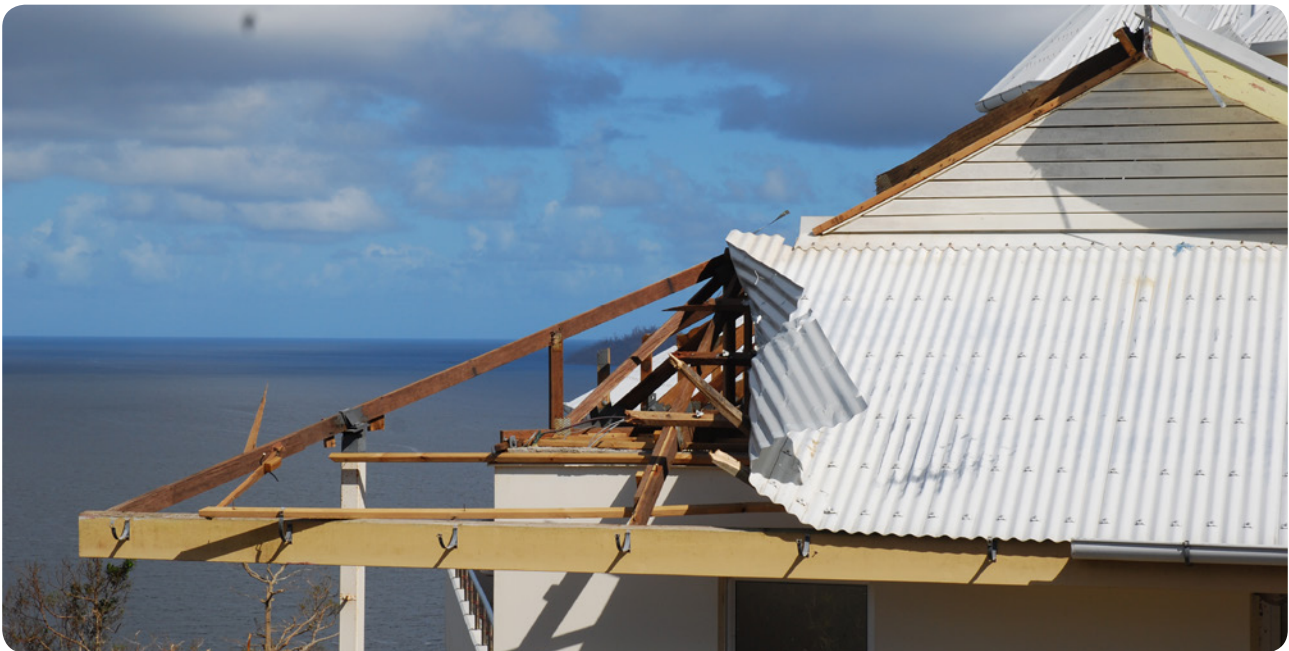
Figure 1.1: Wind damage to houses.
