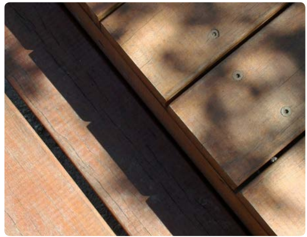
Figure 3.20: Incorrect orientation of boards at landing.
