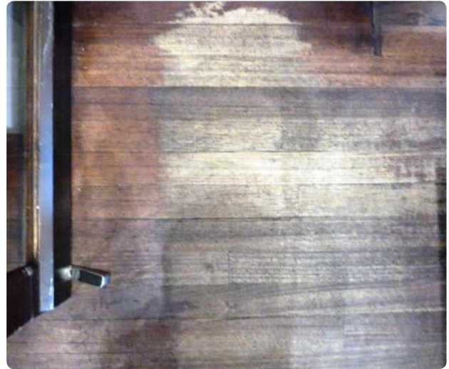
Figure 3.47: Coating degradation due to abrasive wear.
