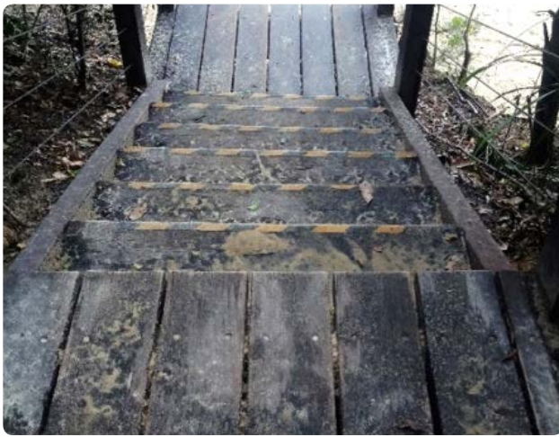
Figure 3.19: Incorrect orientation of boards at landings.
