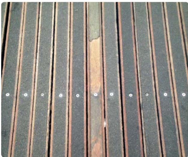
Figure 3.41: Delamination of inset grit-tape straps.
