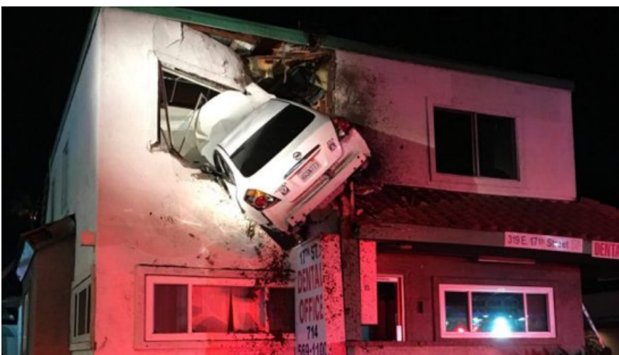
Figure 8.1: Accidental structural damage due to unexpected vehicle impact.
