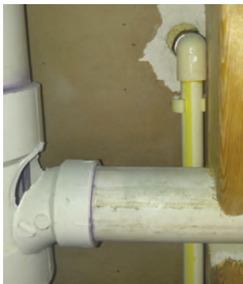
Figure 6.6: Plumbing broken due to axial shortening of the timber frame. (Image is taken from Accommodating Shrinkage in Multi-Storey Wood-Frame Structures Wood Product Council)
