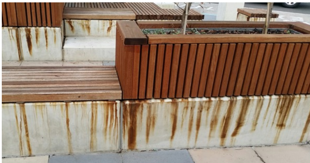
Figure 7: Tannin staining to support structure. (Image: Place holder)
