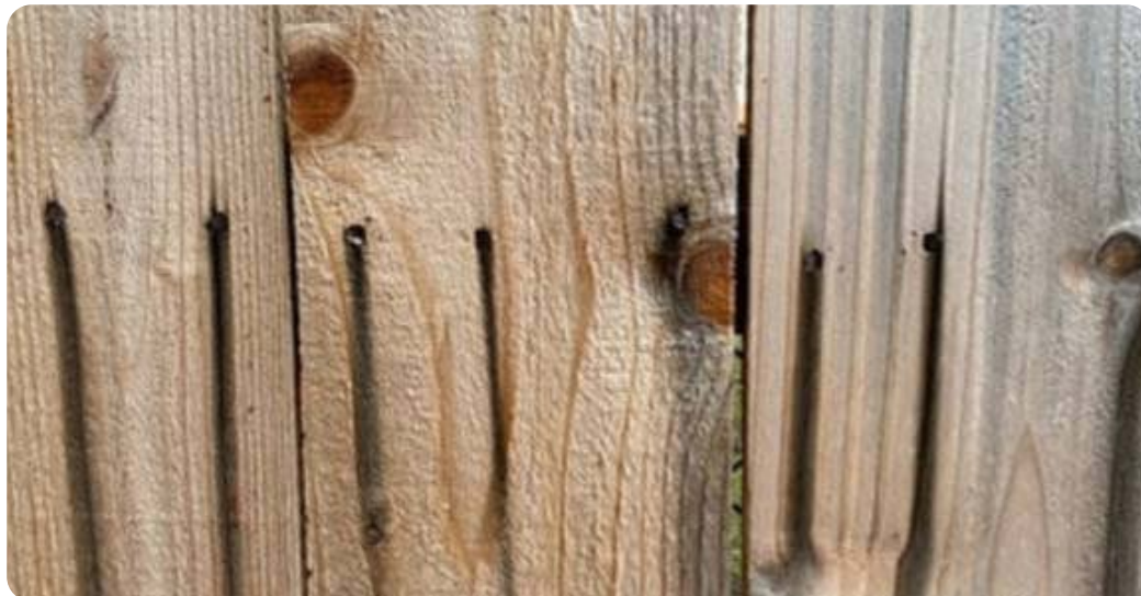
Figure 6: Iron staining on wood from metal nails. (Image: TDA)
