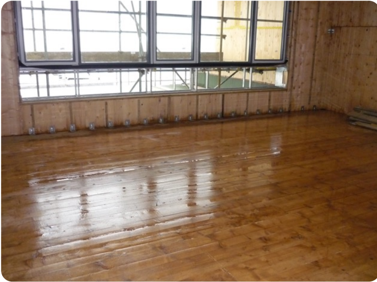
Figure 14: Excessive water on a mass timber construction site. (Image: TDA)
