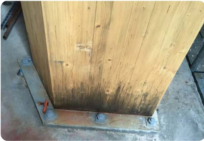
Figure 1: Mould growth on mass timber column (Image credit: TDA)
