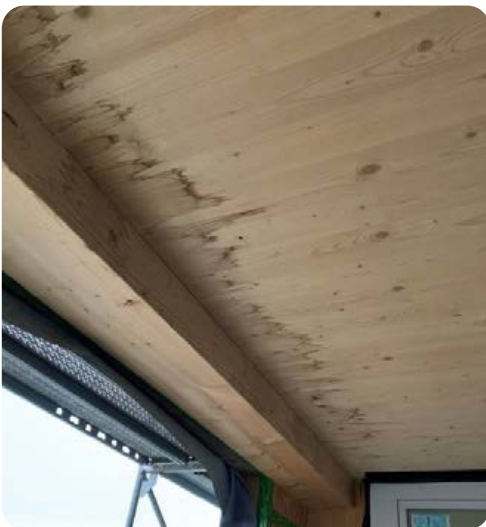
Figure 5: Water staining on the underside of a CLT panel. (Image: TDA)
