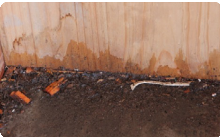
Figure 30: Debris accumulating against a mass timber wall, leading to moisture bypassing end protection. (Image: XLam Australia)
