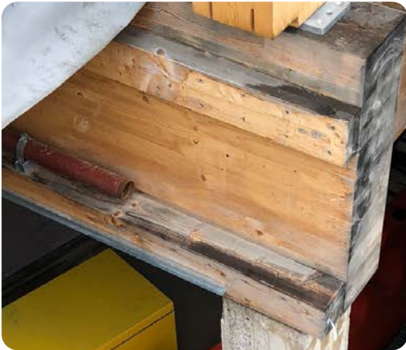
Figure 8: Mould on timber beam. (Image: TDA)
