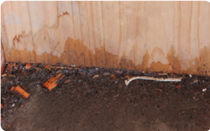
Figure 15: Debris accumulating against a timber wall, moisture by passing end protection. (Image: XLam Australia)
