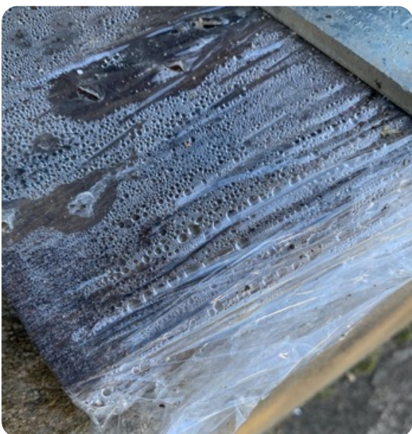
Figure 12: Impermeable wraps without ventilation causing condensation. (Image: TDA)
