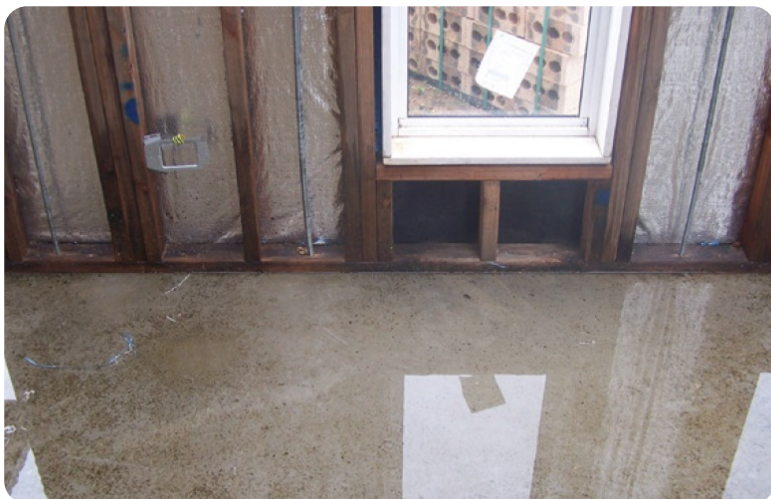
Figure 9: Excessive water on a timber-framed construction site. (Image: WoodSolutions)
