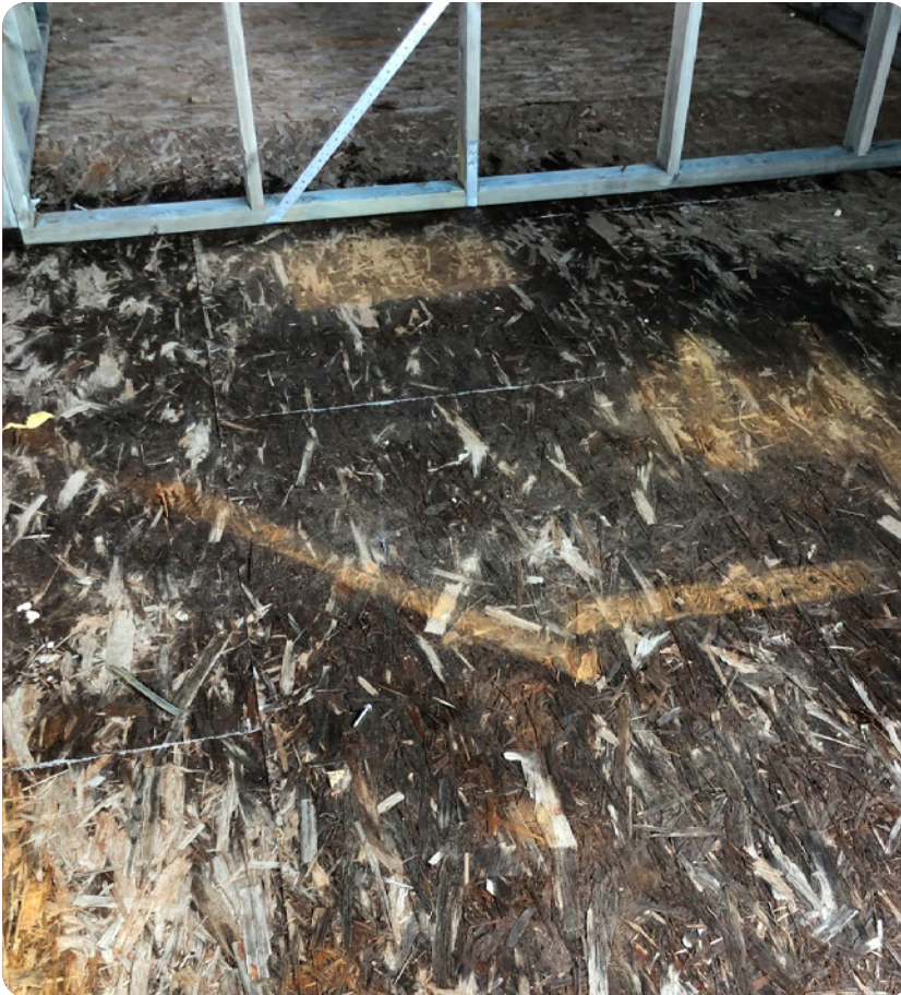
Figure 1: Mould growth on timber frames and sheet flooring (Image: Meyer Timber).
