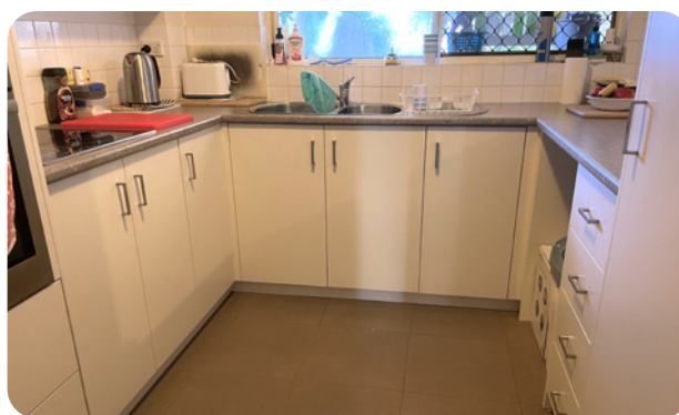
Figure 22b: Two-pack finished high-density fibre board kitchen after a flood (Image Credit: JDA)
