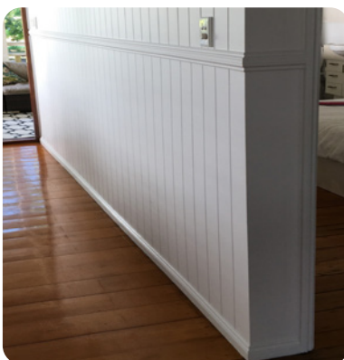
Figure 21b: Fibre-cement vertical joint sheeting with hardwood mouldings and skirting after a flood event (Image Credit: Sedgwick)
