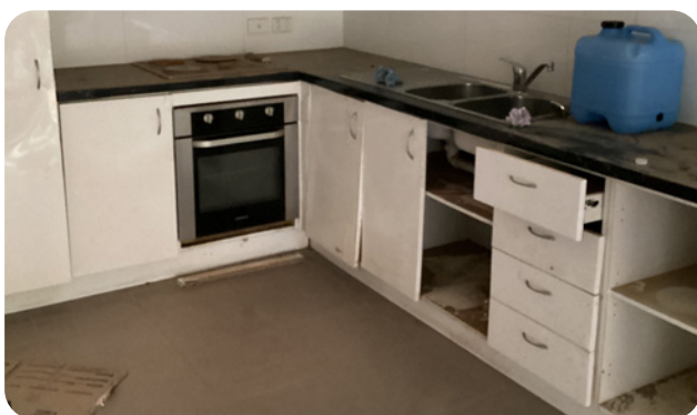
Figure 22a: Laminated medium-density fibre board kitchen after a flood (Image Credit: JDA)
