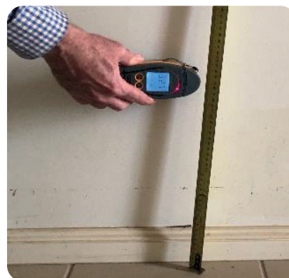
Figure 21c: Plasterboard retains moisture content > 200 mm above flood event. (Image Credit: Sedgwick)
