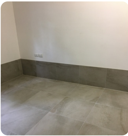
Figure 24a: Tiles with epoxy grout after a flood (Image Credit: JDA)
