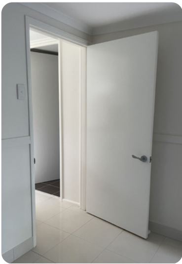
Figure 23: Solid core door after a flood (Image Credit: JDA)
