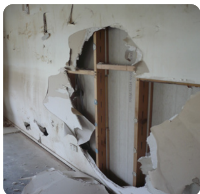
Figure 21a: Plasterboard after a flood event. (Image Credit: Sedgwick)
